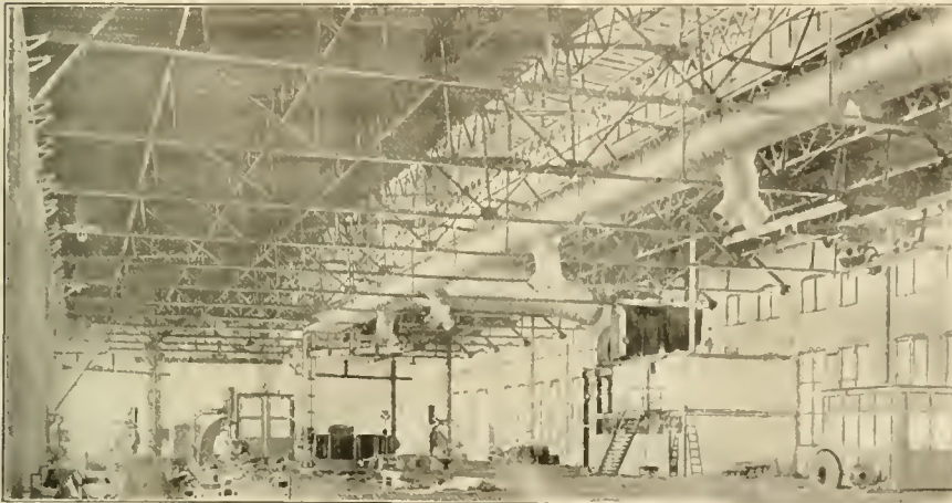
HEATING APPARATUS IN THE SHOPS OF THE CHICAGO, ROCK ISLAND & PACIFIC RAILWAY.
